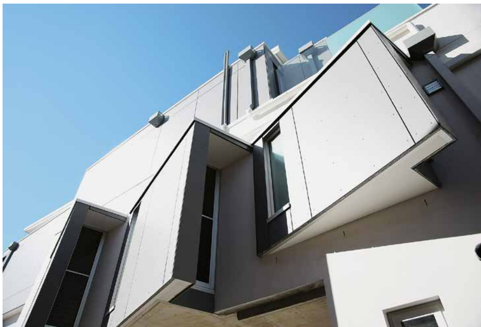
The combination of a façade in cement composite panelling and glass louvres make for a well lit and ventilated structure, sustaining the harsh marine climate.
